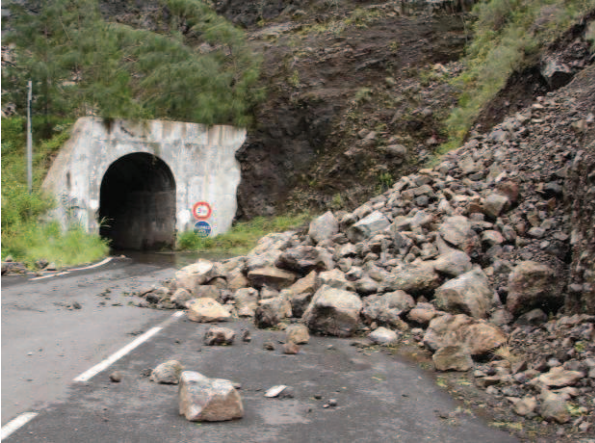
Eboulement - RN5, tunnel P. BOTH (Gamède, 2007)
